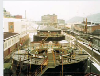
Industrial wastewater treatment, Czech Republic Realization: 1995 Location: Spolchemie, Ústí nad Labem Capacity: 90 000 PE
