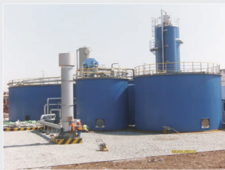
Industrial wastewater treatment plant, Russia Realization: 2016 Location: Vladivostok Capacity: 6 pcs. tanks
