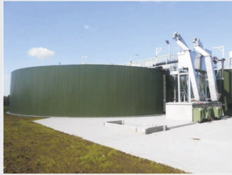
Waste water treatment plant, Poland Realization: 2015 Location: Wierzbna Capacity: 4 000 PE Purpose: Complete delivery wastewater treatment plant Model: HYDROVIT®SI
