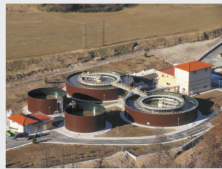
Waste water treatment plant, Bugarska Realization: 2016 Location: Panagurišće Capacity: 19 000 PE Purpose: Complete delivery wastewater treatment plant Model: HYDROVIT®P
