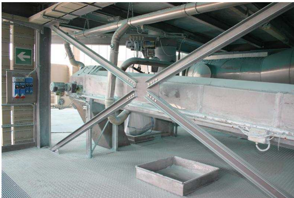
Samec drive station Belt conveyor TN650
