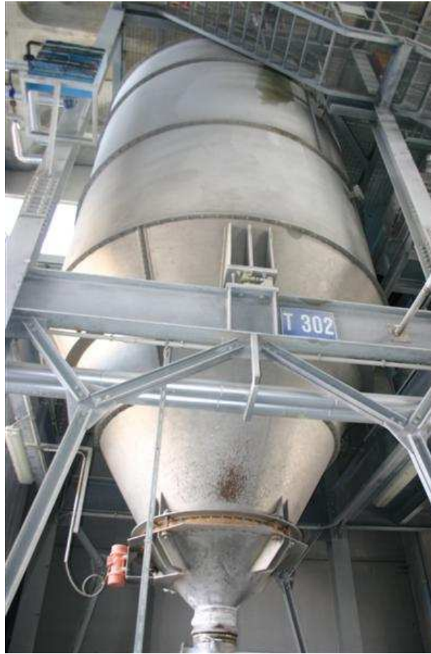
Urea silo storage 130 m 3 capacity
