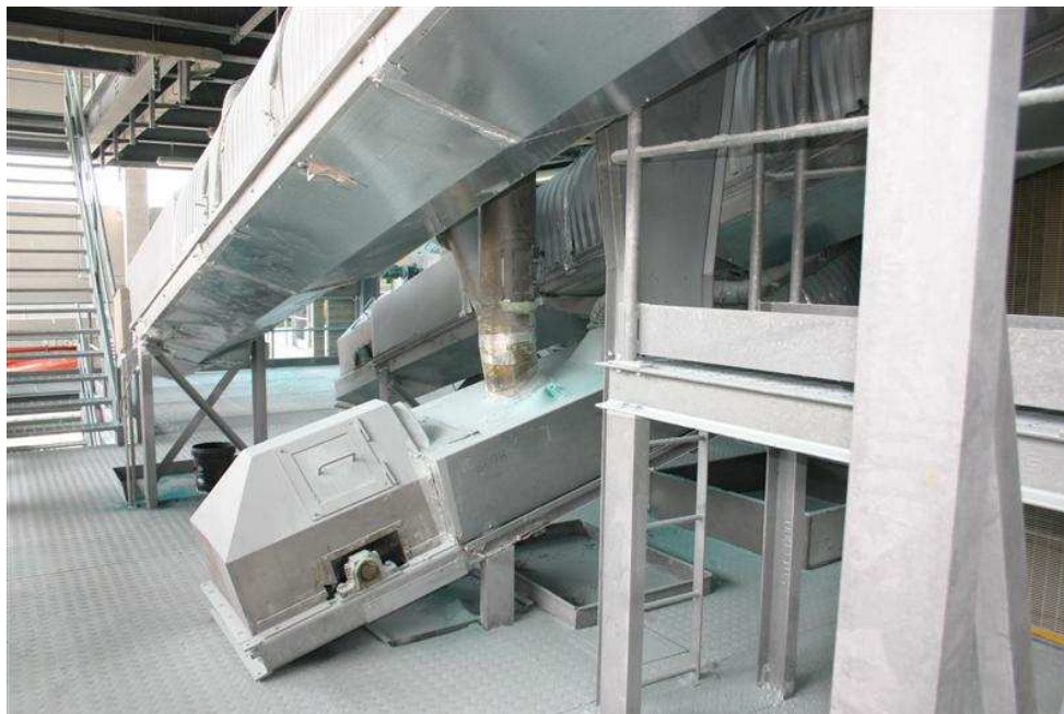
Samec return station Belt conveyor TN650
