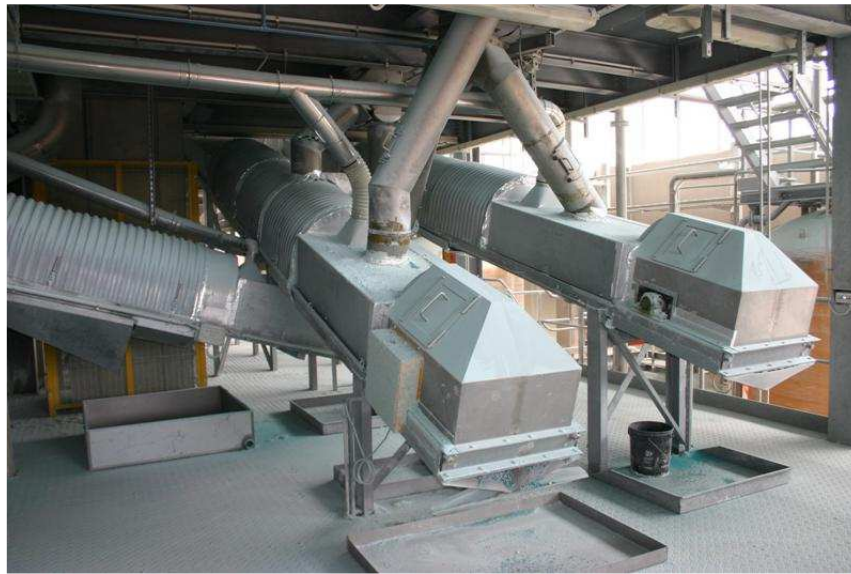
Samec Belt conveyor TN650 – de dusting system
