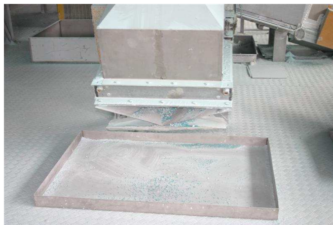
Samec Belt conveyor TN650 – tank under return station
