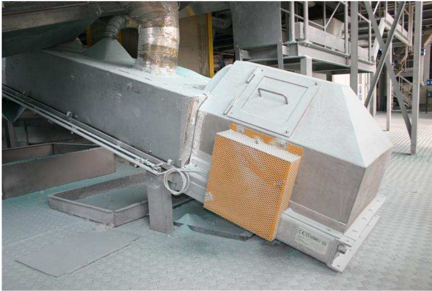
Samec return station Belt conveyor TN650
