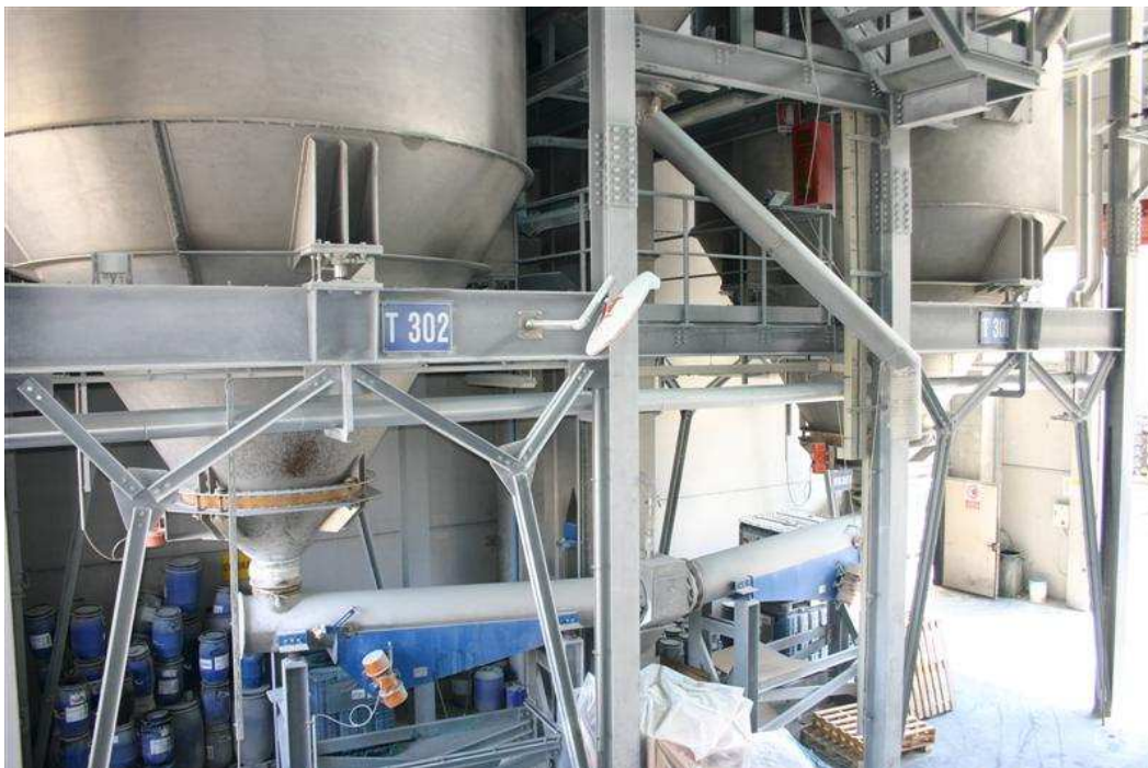
Urea silo extracting
