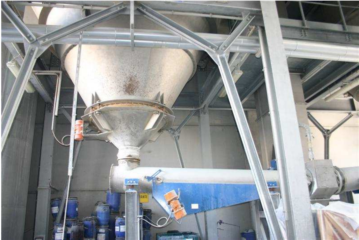
Silo with vibrating bottom extracting
