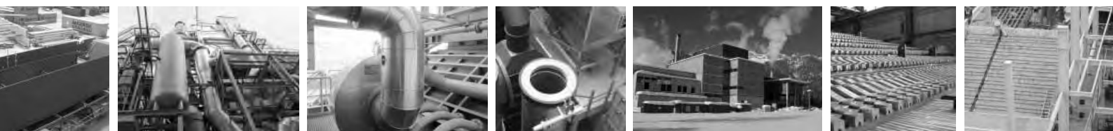
✓ 5 MW thermal oil heater with 1 MW ORC turbine
