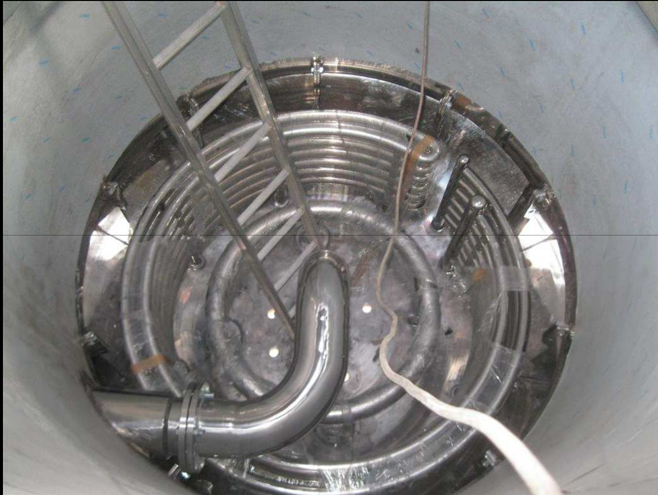
Boiler equipments and Pressure Vessels
