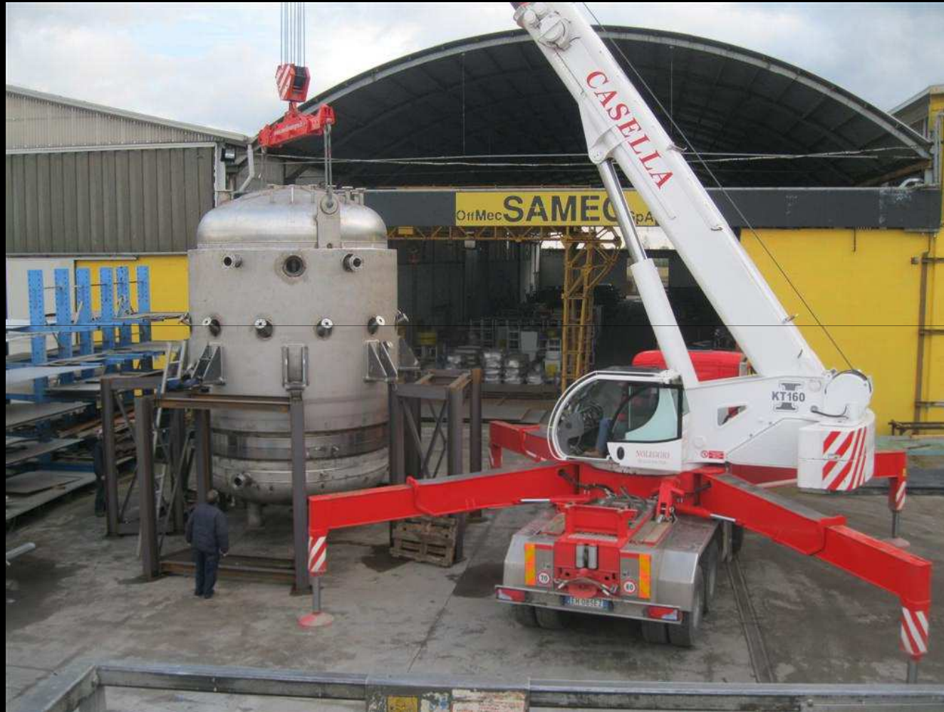
Boiler equipments and Pressure Vessels
